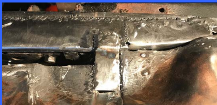
Outer part of the floor pan at the junction being replaced. This required blending it into the new side panels with the new beam acting as the common connection point.
