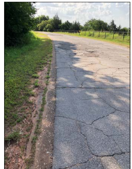
Here is a stretch from the Model A era, concrete-lined road with curbing.
